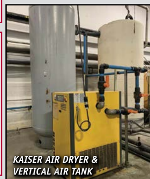
2015 KAISER ROTARY SCREW AIR COMPRESSOR, 50 H.P.
