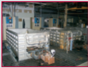
MORTON BEAM DYE MACHINES
