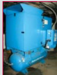
QUINCY AIR COMPRESSOR
