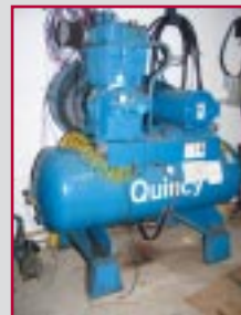
QUINCY AIR COMPRESSOR
