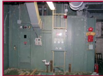
DUST COLLECTION SYSTEM
