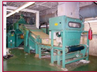
COMPUTERIZED CONVEYOR SYSTEM
