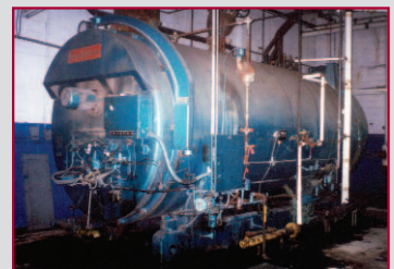
CLEVER BROOKS BOILER
