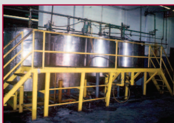
S.S. MIXING TANKS
