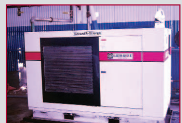
GARDNER DENVER COMPRESSOR
